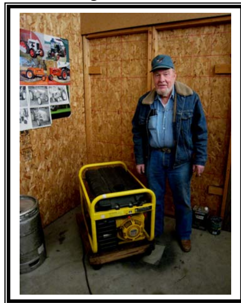
Lion Glenn Dales stands beside our new generator - what a beauty (the generator)
